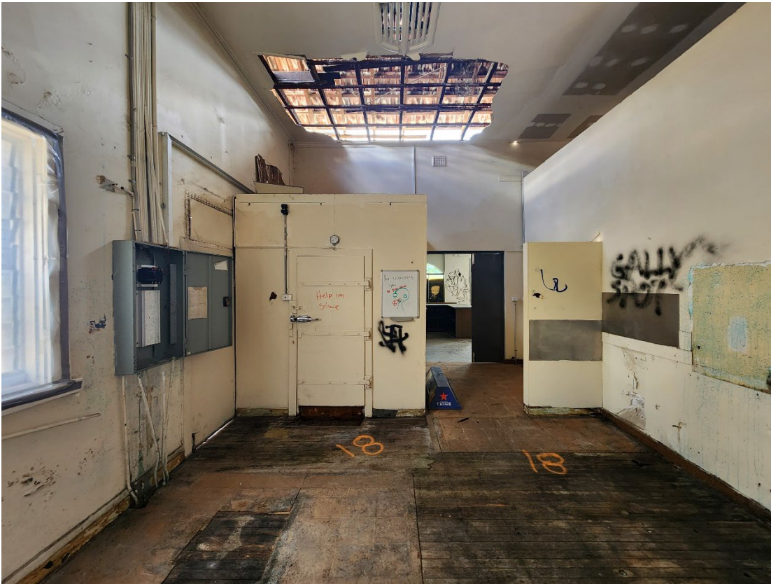
View 29 Timber flooring in the back of house area adjacent to the Kitchen
