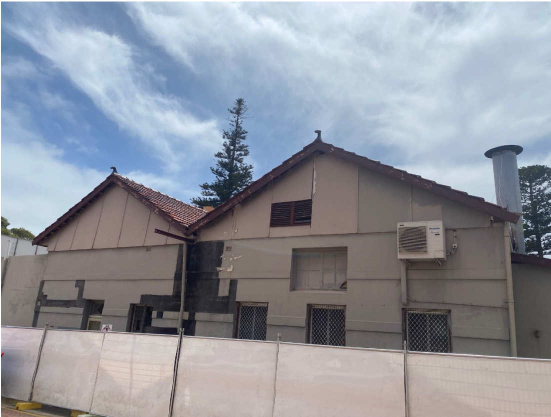
View 23 Western elevation prior to recent removal of asbestos cladding to gables Courtesy Emirge, February 2024
