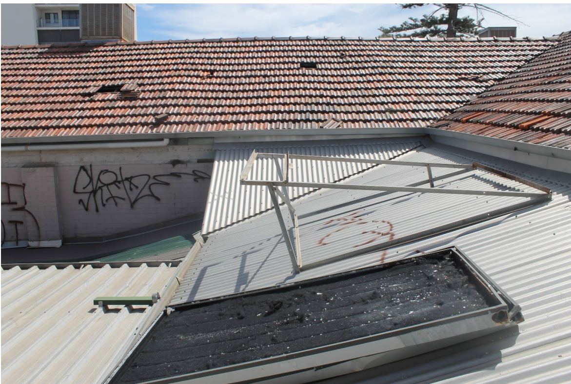
View 100 Configuration of the skillion metal roofing and tiled hipped roofs above the Bar, Saloon and Lounge
