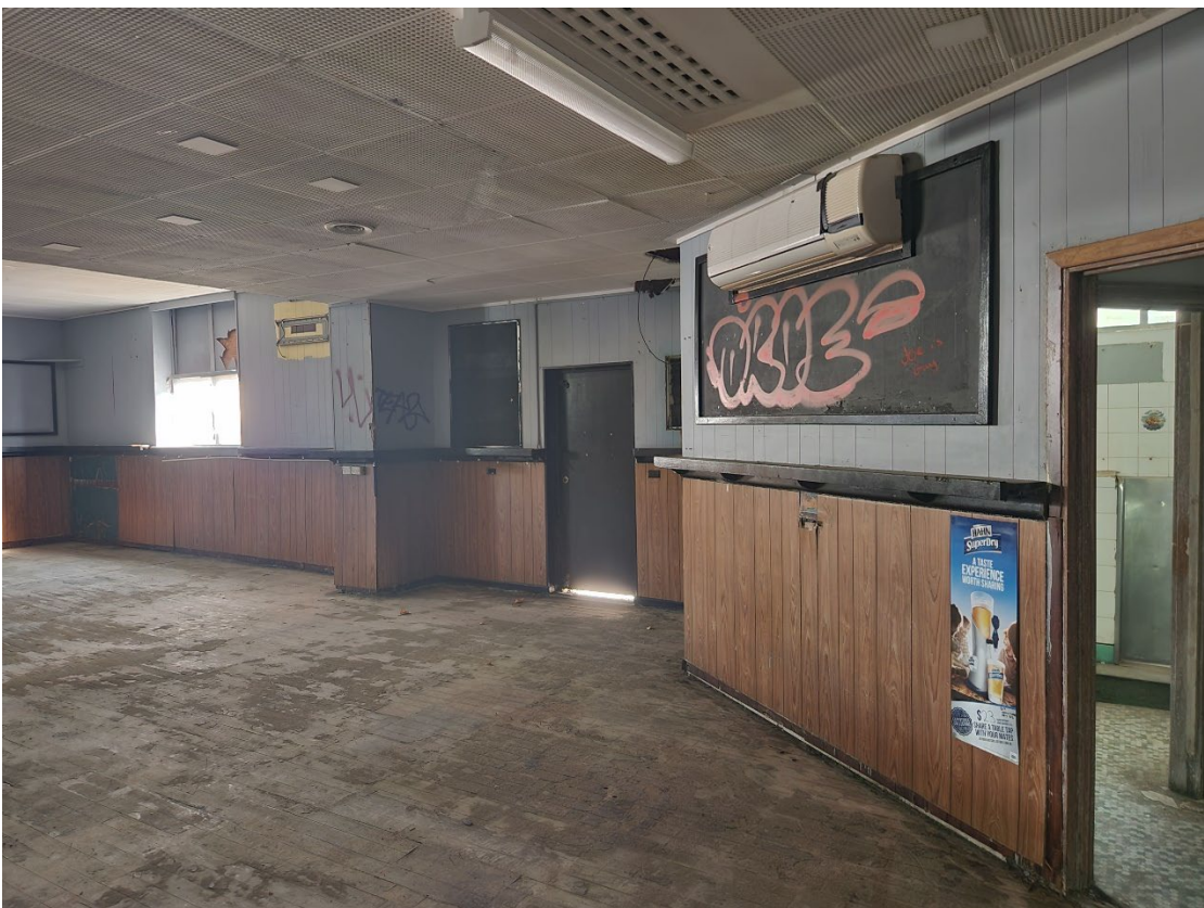
View 60 Access to the toilets of the Bar on the far right and timber dado detail along the walls
