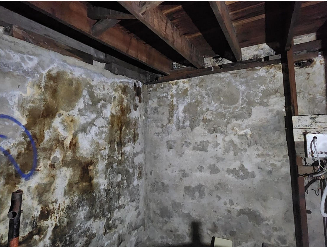
View 105 Plastered walls in the basement under the oldest section of Rockingham Hotel
