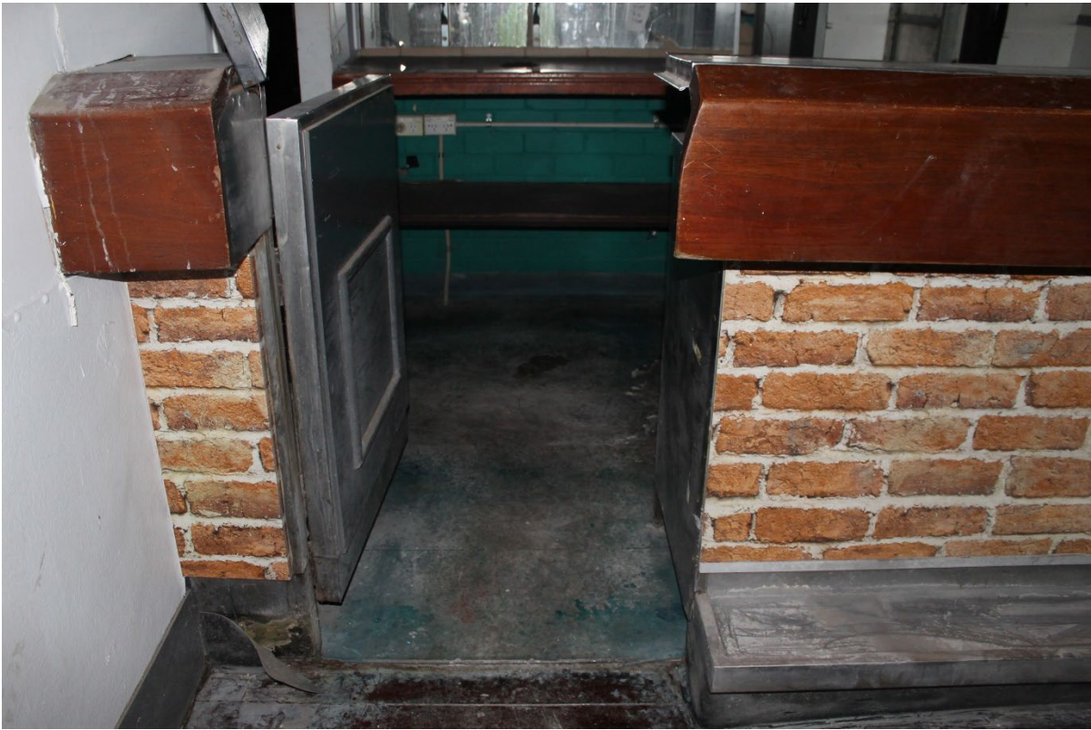
View 39 Detail view of access behind the counter in the Dining Room
