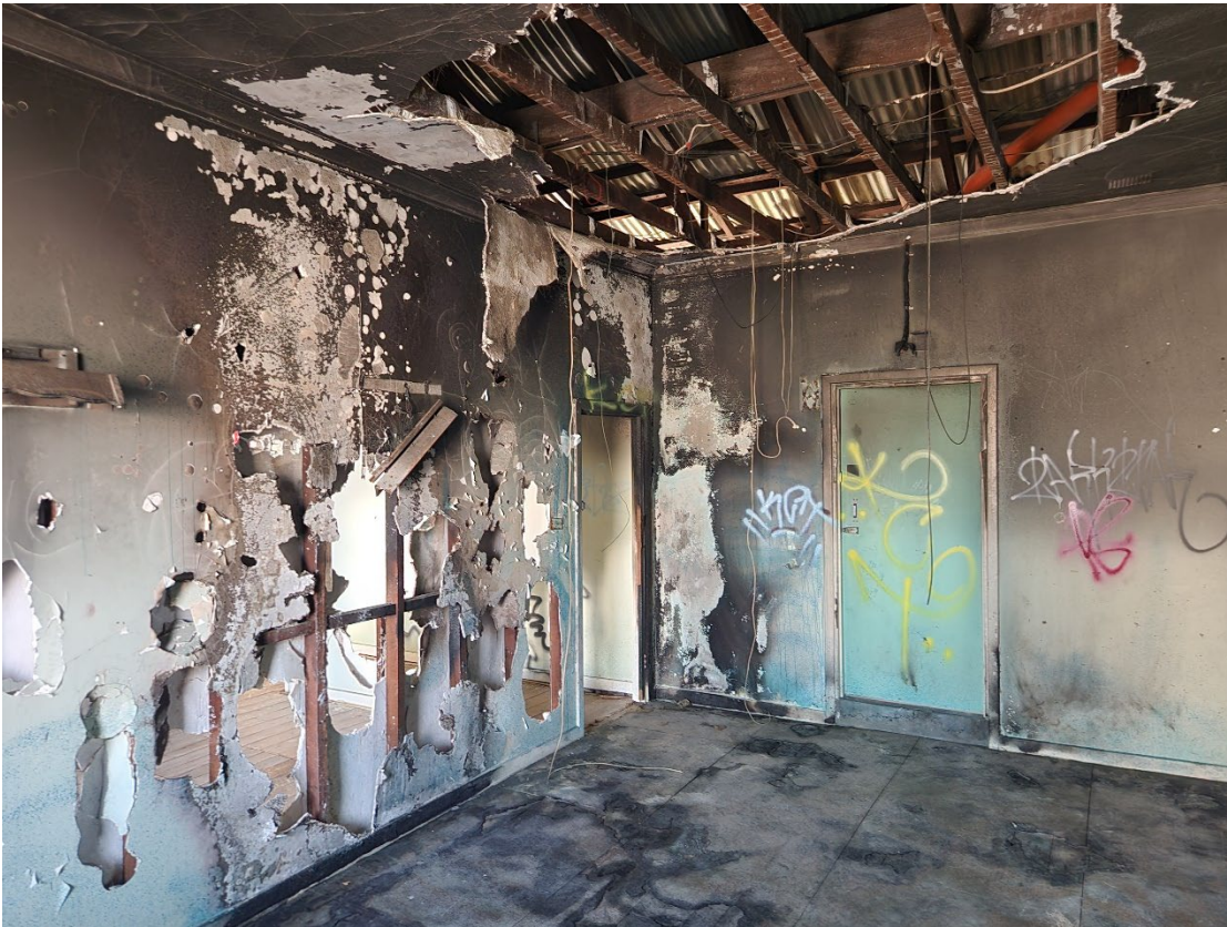
View 73 Recent damage to plasterboard walls in the Lounge
