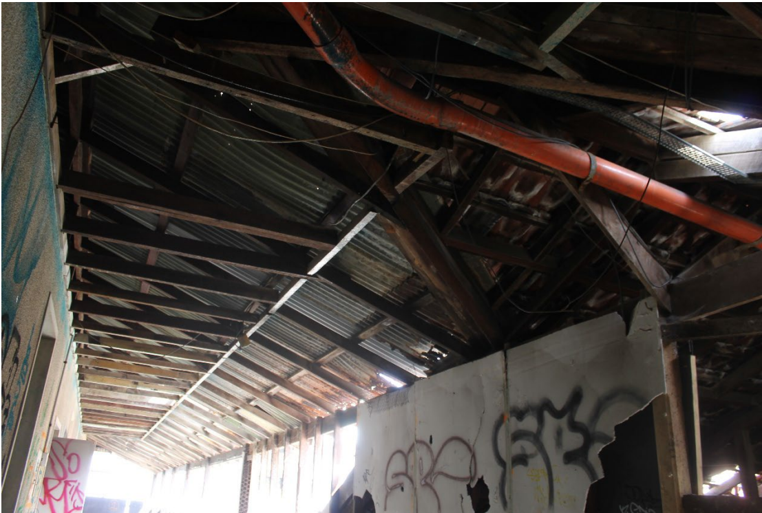
View 97 Timber roof structure over verandah (linings removed during recent asbestos clearing works)
