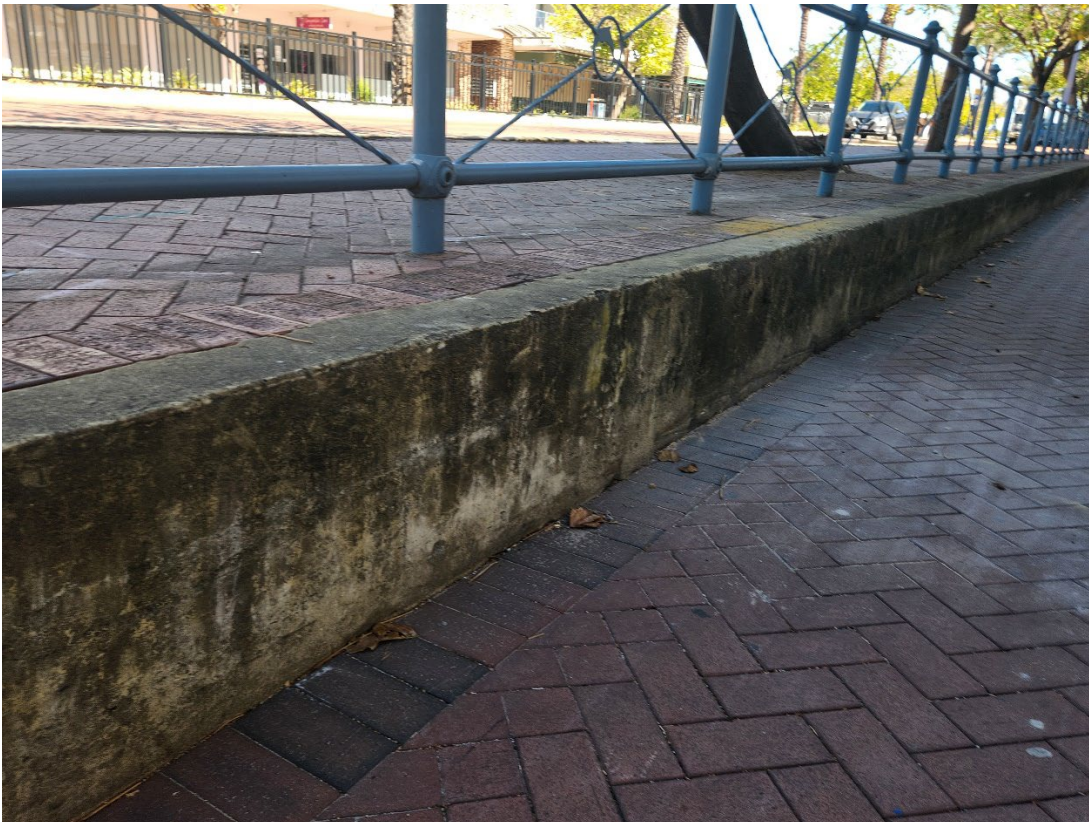
View 10 Level difference between pedestrian footpath and building apron along Kent Street
