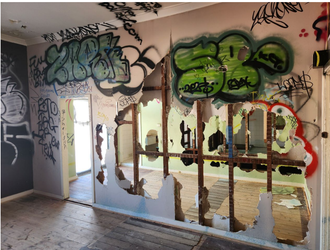
View 80 Room 2 interior with timber floorboards and recently damaged walls
