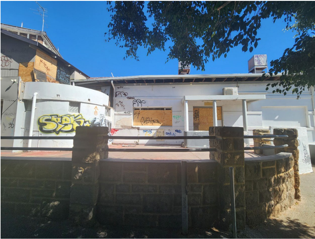
View 17 Vuggy limestone retaining walls with metal handrails to the outdoor area outside the Lounge
