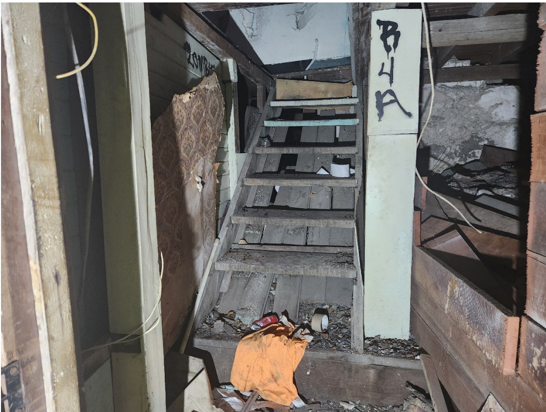
View 111 Steps from the basement leading up to the trap door in the Kitchen
