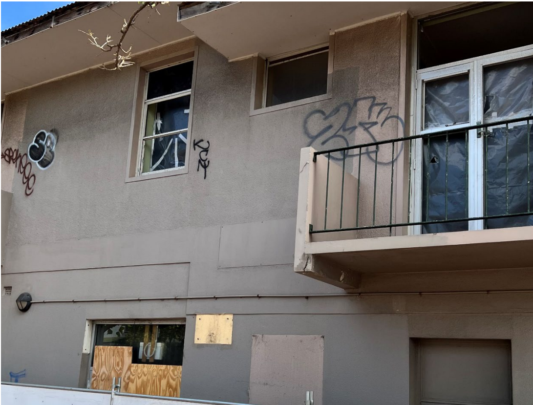
View 21 Close up view of rendered walls with paint finish on the southern elevation
