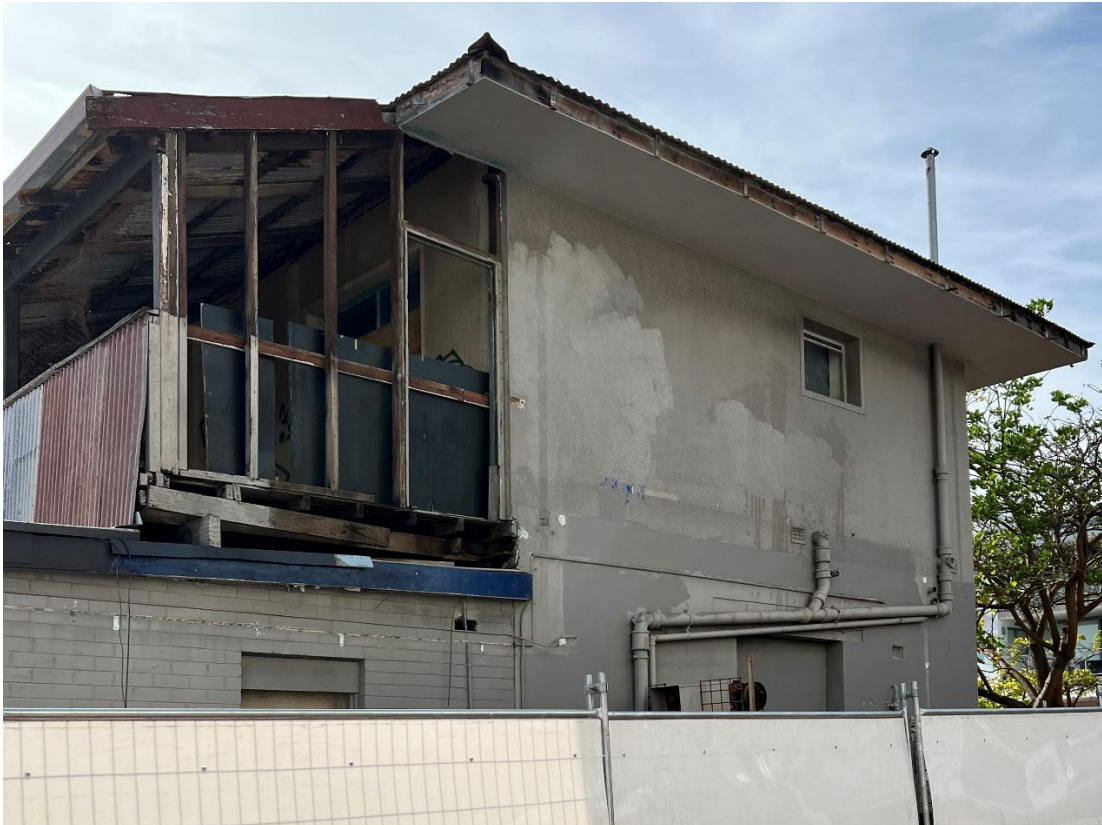
View 24 Upper section of the oldest part of the building following recent removal of asbestos cladding to verandah
