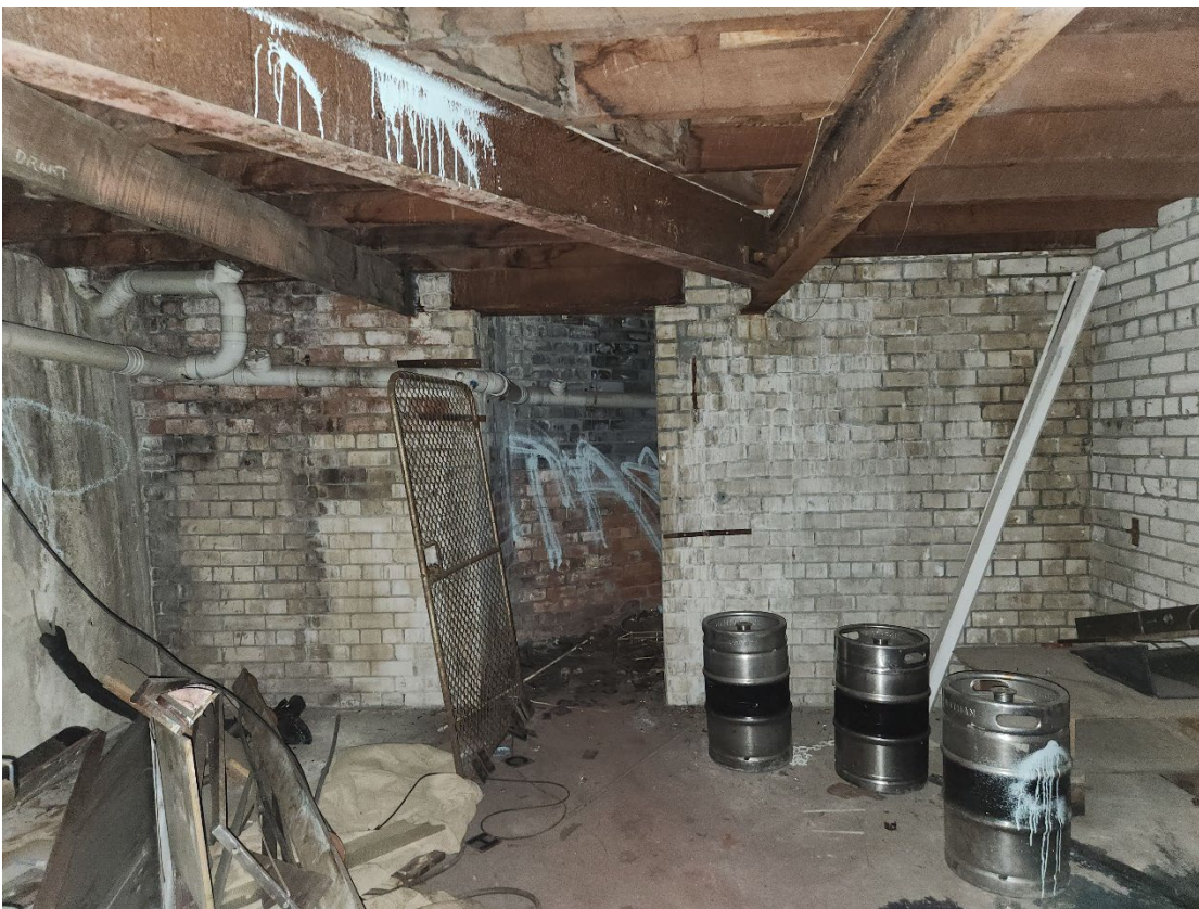
View 106 Brick walls in the basement with steel beam supports to the floor above
