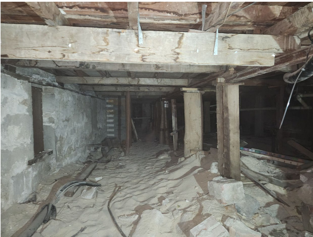
View 113 Crawl space in the basement with timber stumps, bearers and joists supports
