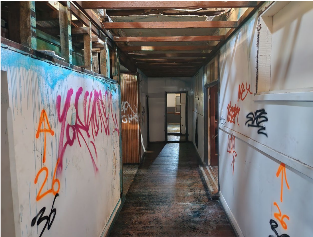
View 47 Corridor off the Lounge (asbestos containing linings removed recently)
