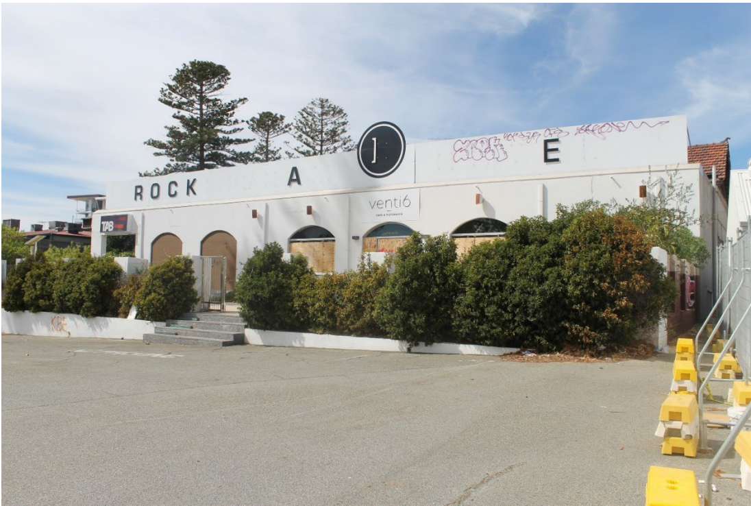
View 11 Northern elevation of Rockingham Hotel with remnant individual lettering signage and hoardings following asbestos removal
