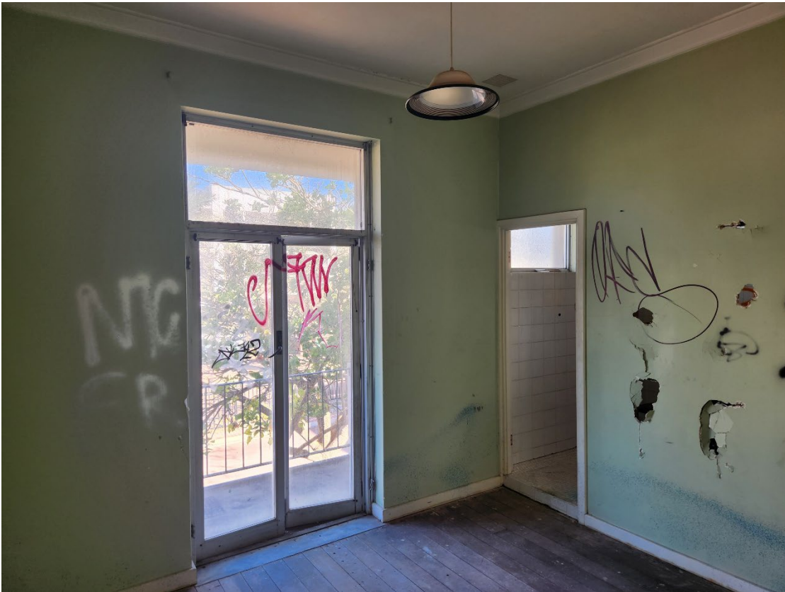
View 86 Metal framed door and fanlight in Room 5 leading to the balcony
