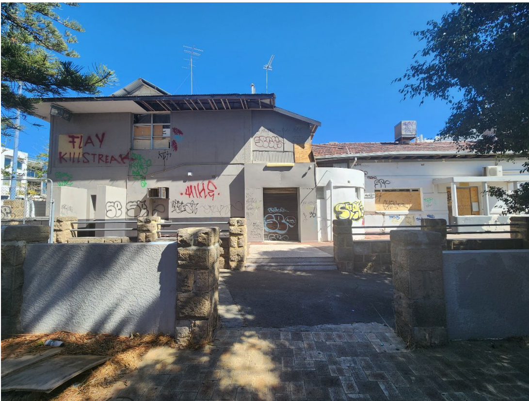
View 16 East elevation of Rockingham Hotel with some cladding removed during recent asbestos removal
