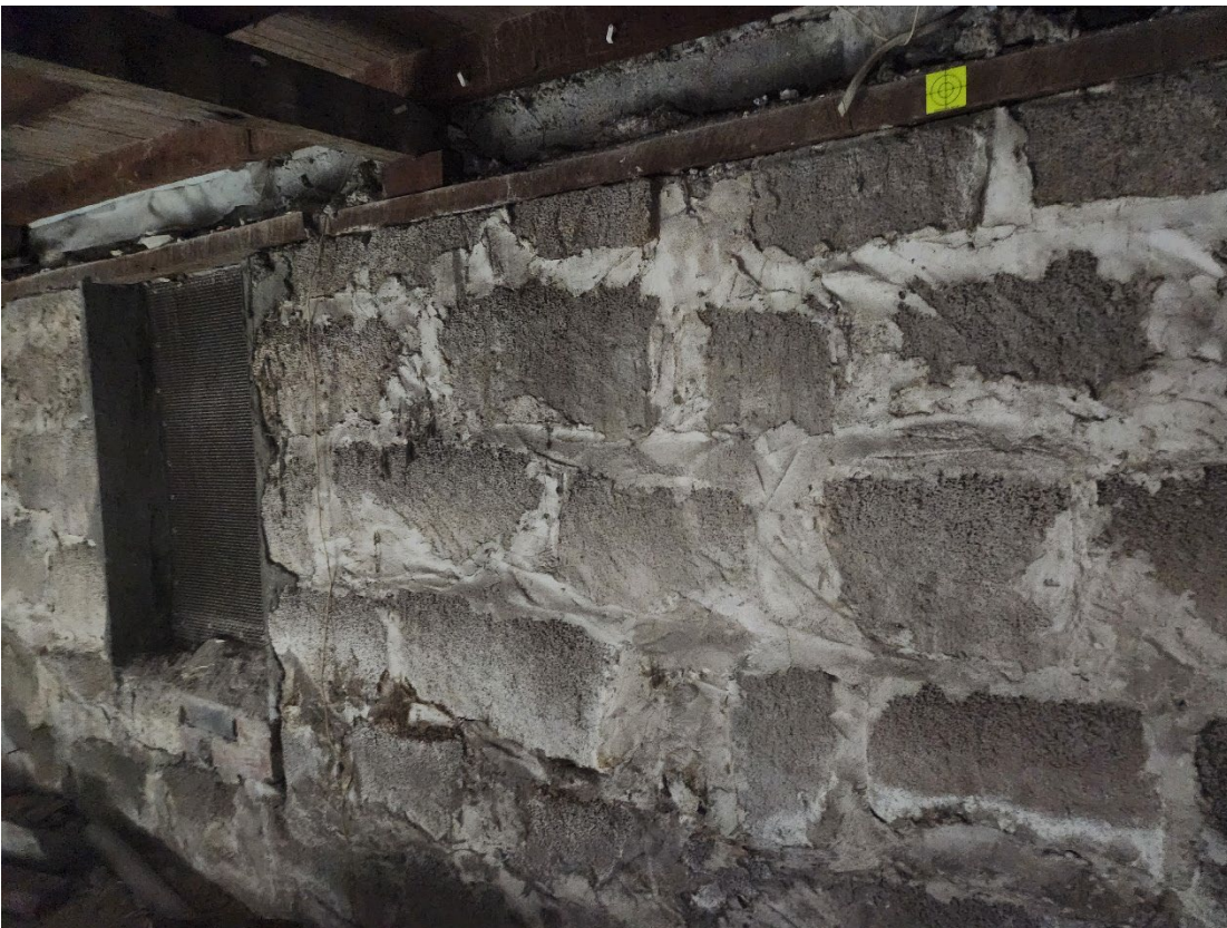
View 113 Sealed tunnel at the northern end of the basement inserted in vuggy limestone blocks
