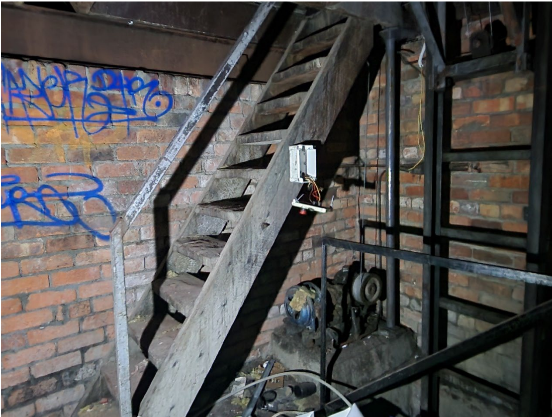
View 109 Detail of timber steps and metal handrail access into the basement from the bar area
