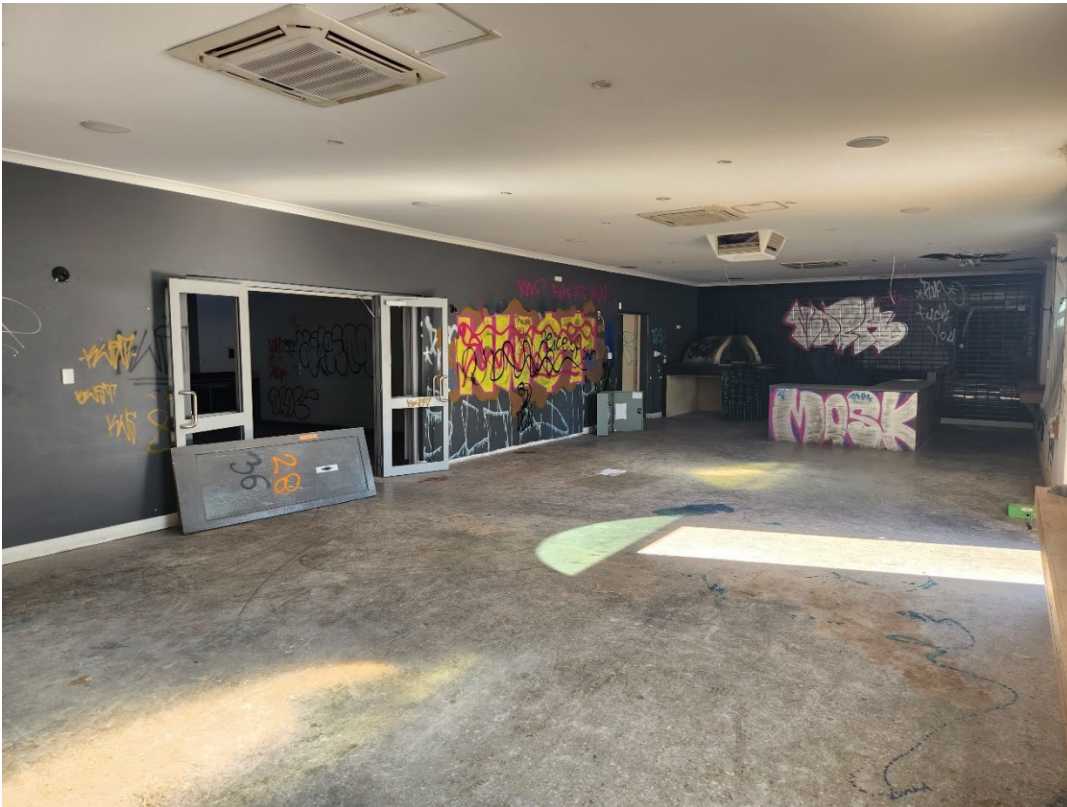
View 25 Function room with concrete flooring and service counter in the background
