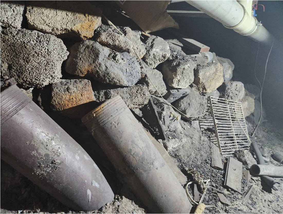
View 113 More rubble and redundant fixtures under the basement
