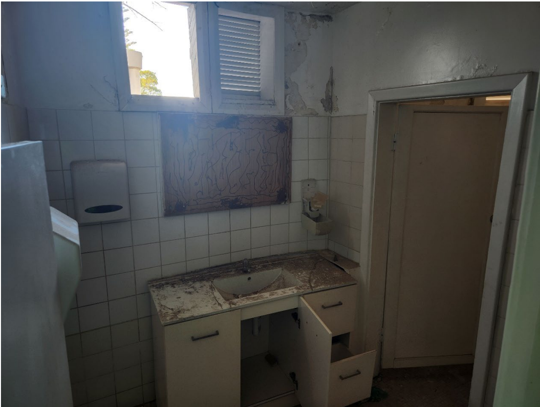
View 49 Female toilet with timber louvred windows along curved section of wall
