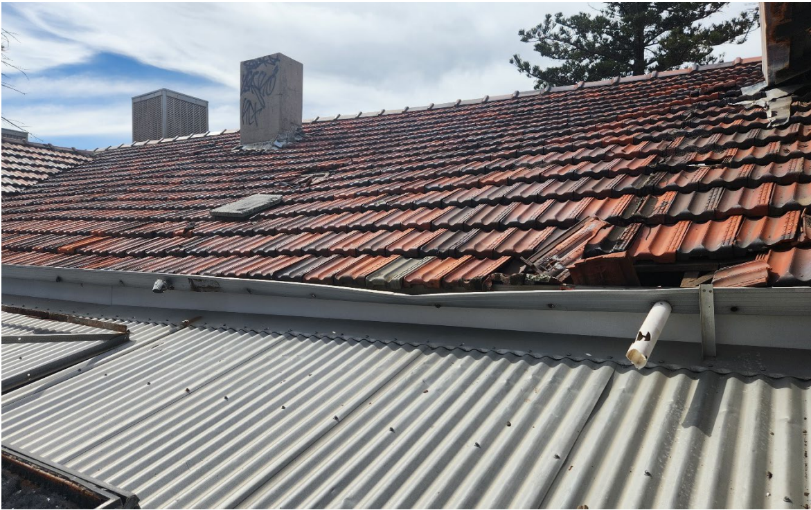
View 99 View of the tiles and corrugated metal roofing over the Ground Floor structure as viewed from the verandah on First Floor
