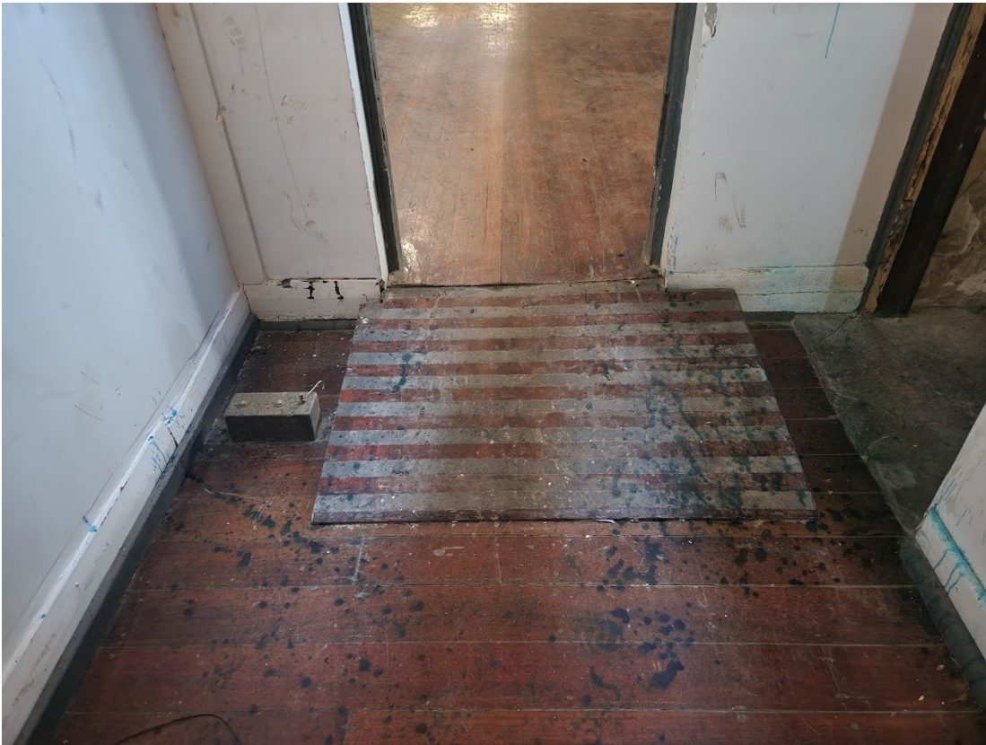
View 46 Ramped access covering the step down into the passage way off the Lounge
