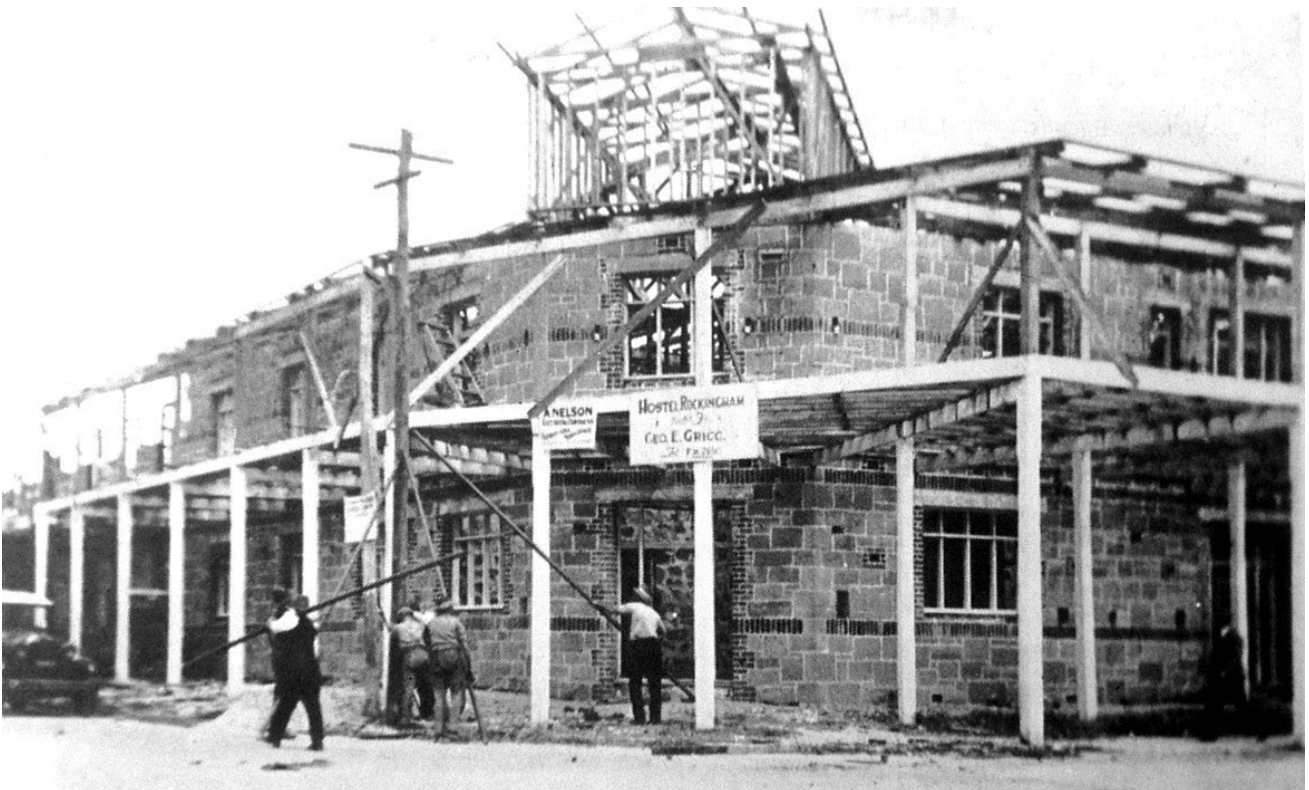
Figure 20 Hostel Rockingham construction, 1935-36 Courtesy Draper & Kerford, Rockingham from Port to City 1888 , p. 59
