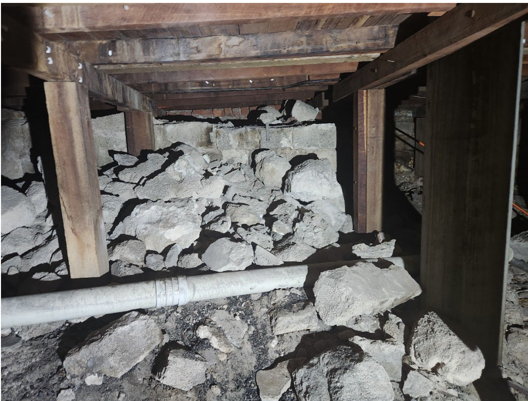
View 113 Rubble stones under the later part of the basement with timber stumps supporting the Ground Floor
