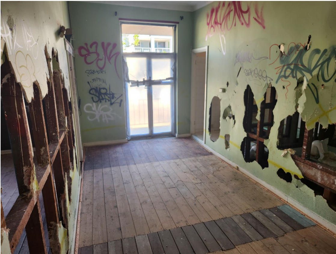
View 81 Timber floor boards in Room 3; access to balcony in the background
