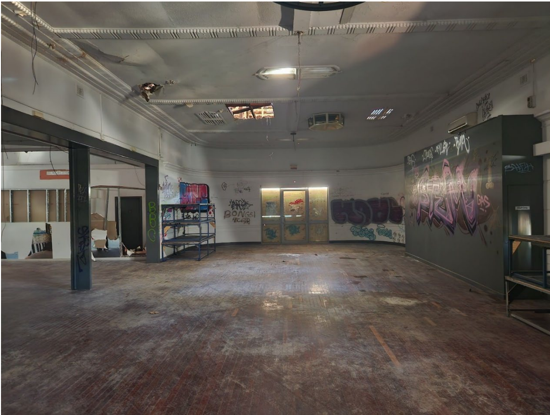
View 43 View of the Lounge with decorative detail in ceiling and curved walls in the background
