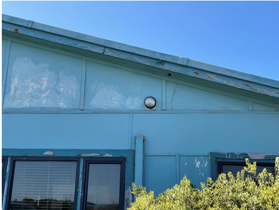
Figure 17: Damaged fibro panelling to gable element and damaged timber fascia
