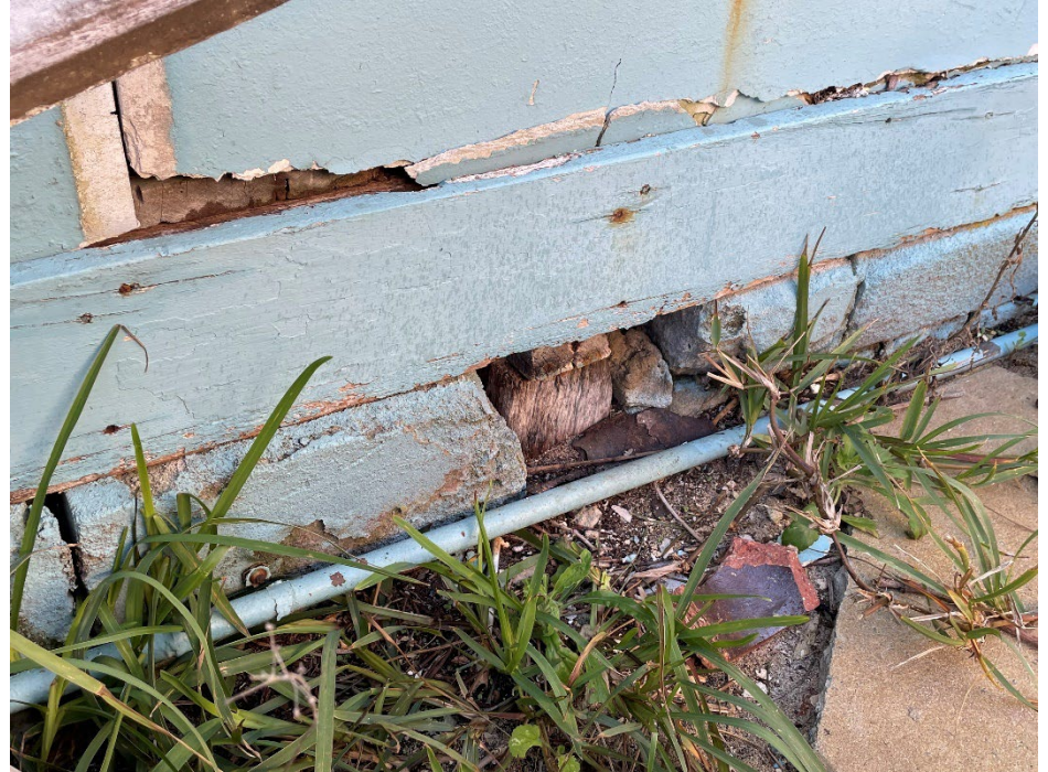
Figure 16: Damaged fibro panelling
