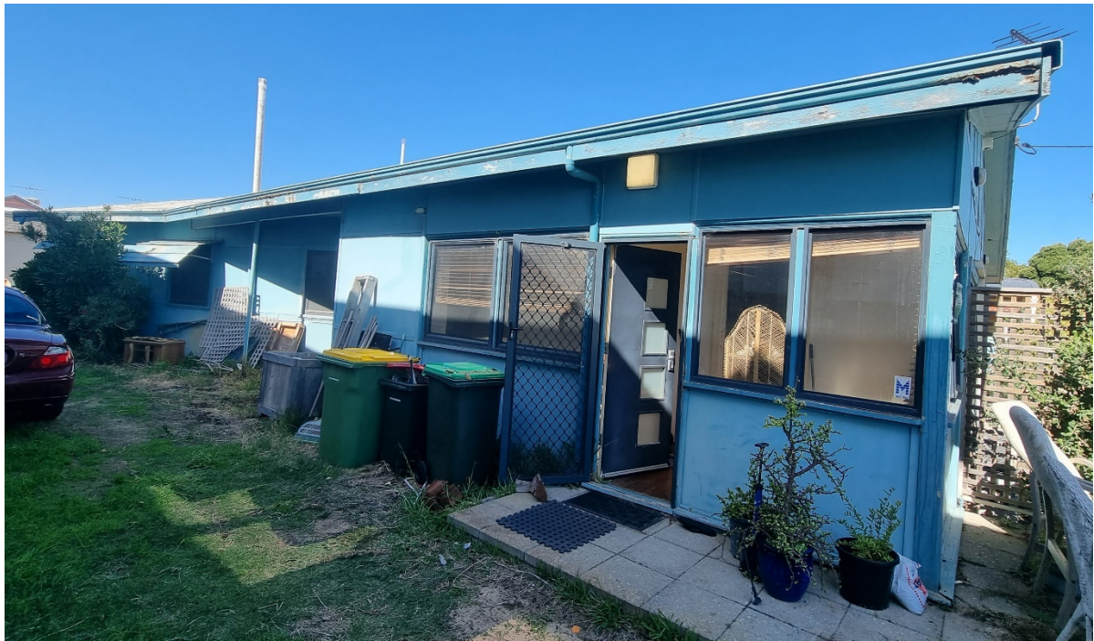
The side elevations are a mix of windows of different dimensions, some with metal clad awnings above and fibro panelled walls. None of the windows or doors are original.
