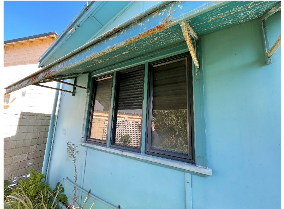
Figure 20: Rusted window awning and replacement windows
