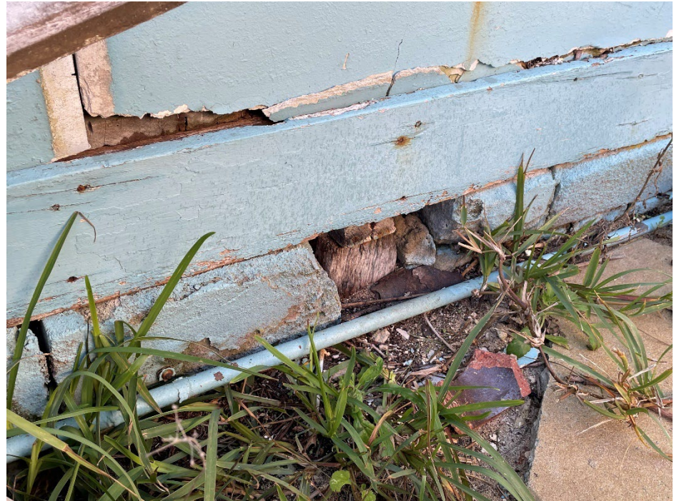
Figure 14: Damaged fibro panelling
