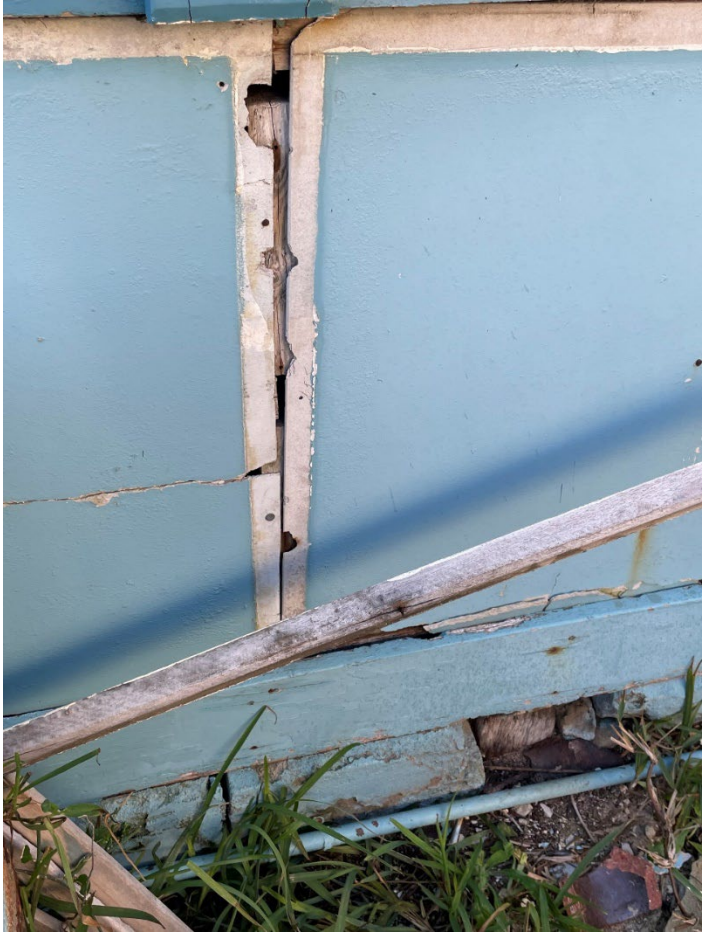
Figure 15: Damaged fibro panelling, missing cover battens
