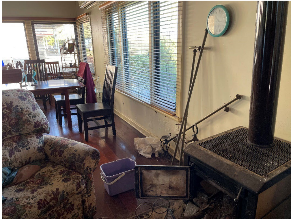
Figure 23: Damp below the windows
