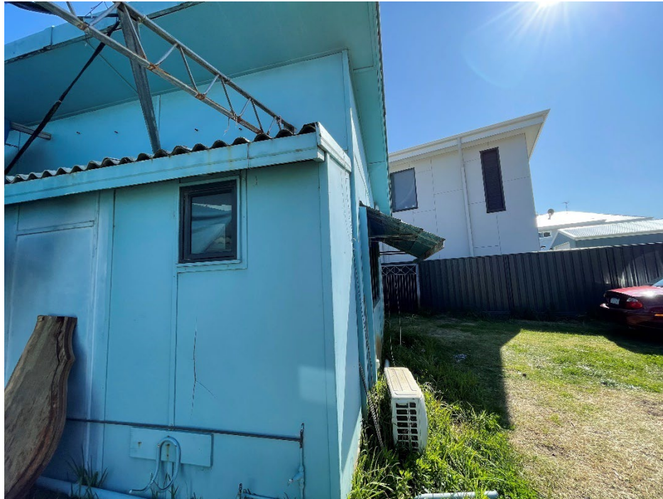
Figure 19: Damaged fibro panelling
