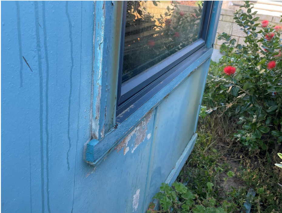
Figure 13: Damaged fibro panelling
