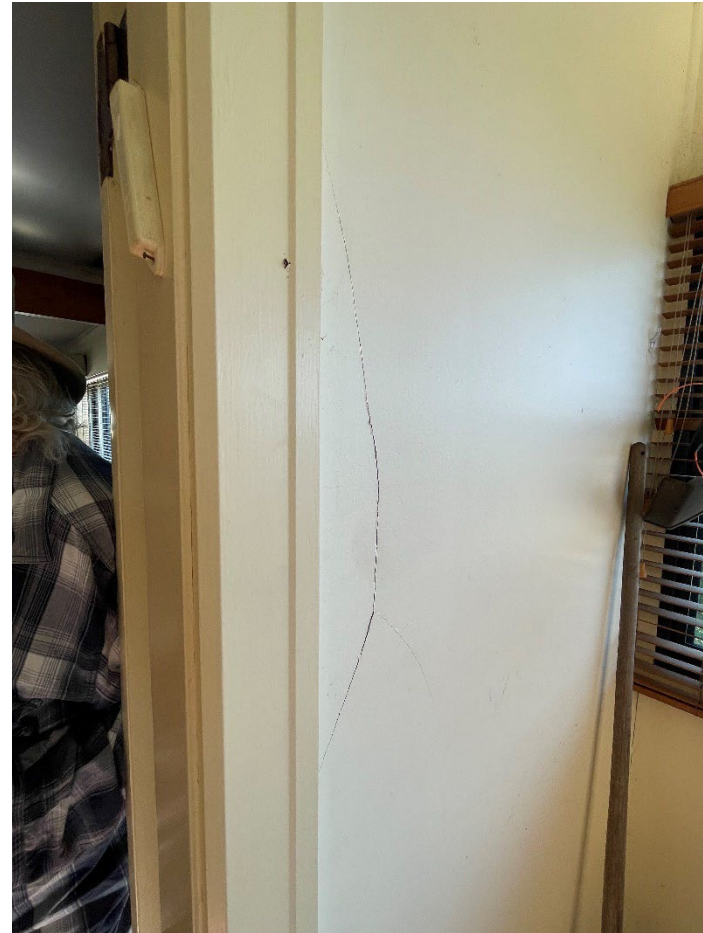
Figure 22: Damaged fibro wall to the interior
