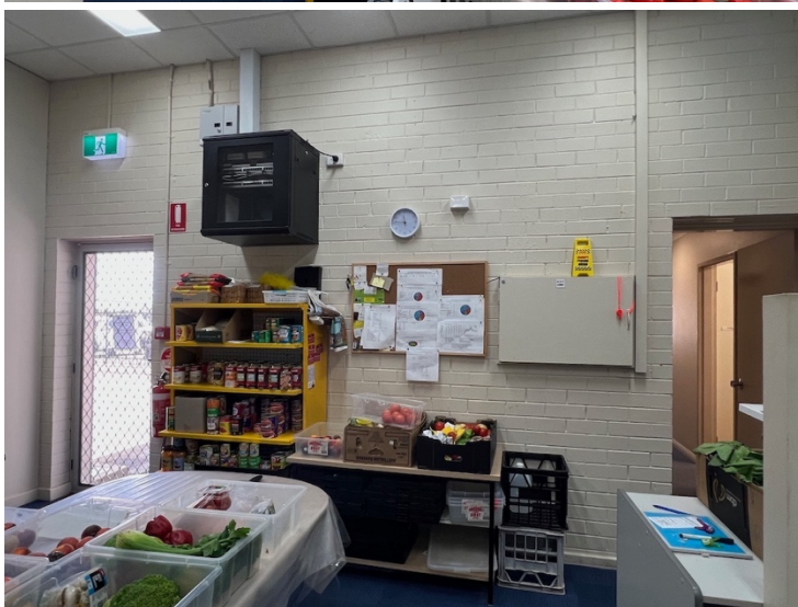
Interior views looking to the south wall, and the northwest corner, at west end of the former appliance room.
