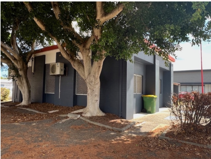
Views looking southeast from the Medical Centre carpark, front showing the Medical Centre (right), and the southeast front corner of the Appliance room. It also shows the impact of the mature trees in close proximity to the building and carpark causing upheaval to the bitumen and kerbing, and likely the foundations of the south wall of the former appliance room.
